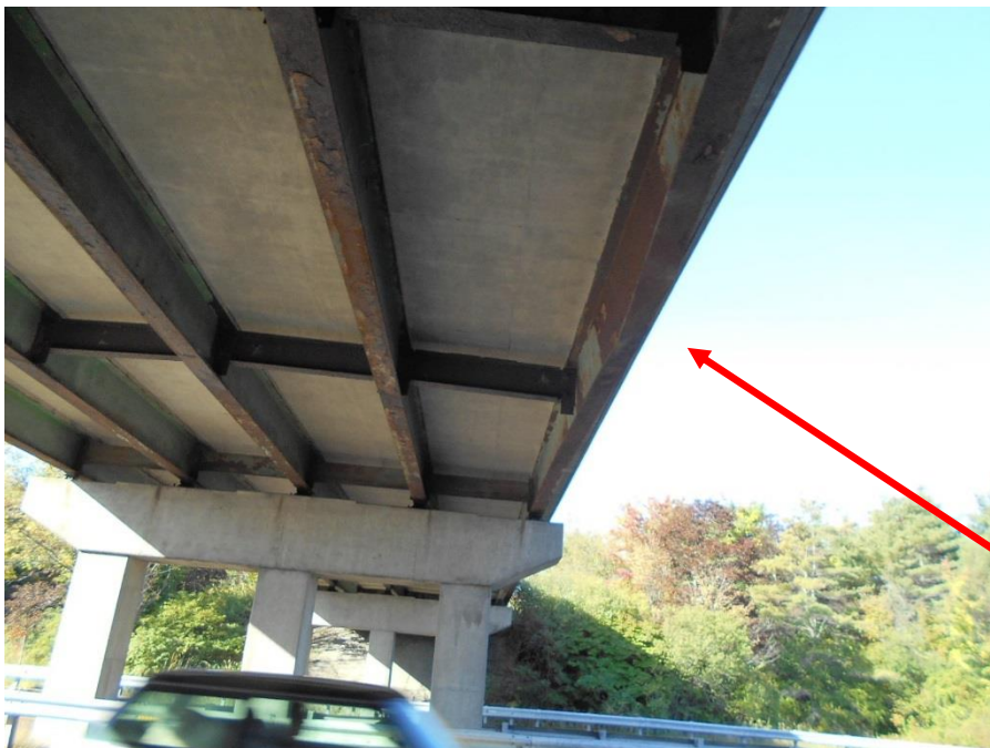
4" plus sweep in northerly exterior beam
